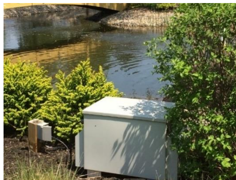
Cabinet installed near pond and electrical power outlet
