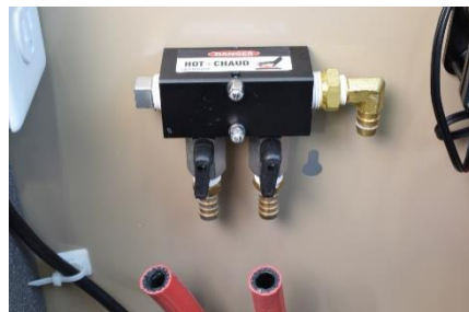
Manifold before connections
