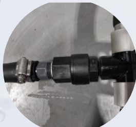
Connection with the feeder line
