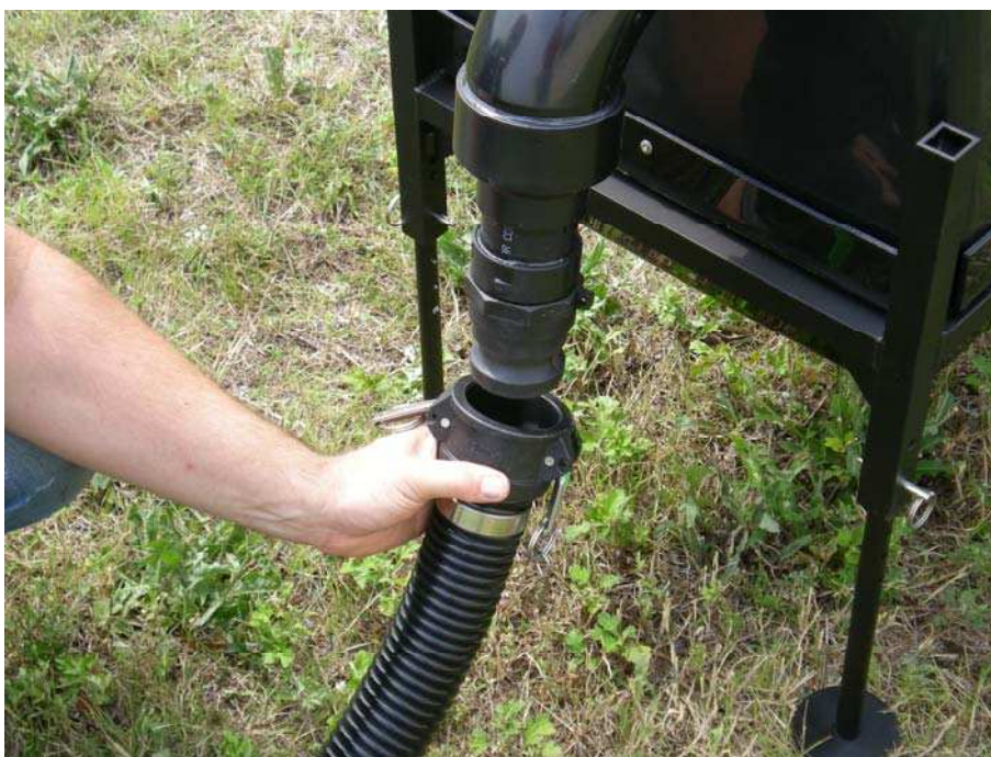
Figure 4 Preparing to install the 2 inch quick connect hose to the filtration unit.
